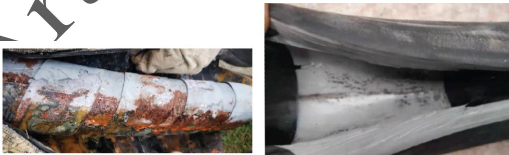
Fig. 5. Examples of failure damages appeared at MV cable accessory interfaces due to multi-physical stresses combined with water ingress [33]
