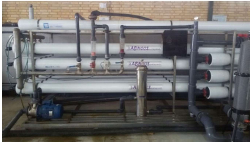
Fig. 1. Membrane system of Sorkheh city treatment plant
